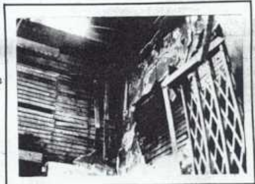
Ceiling and wall where axe was used
